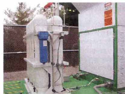
CNG storage bottles at the refueling station built and operated by Clean Energy for Central Jersey Waste’s refuse trucks
